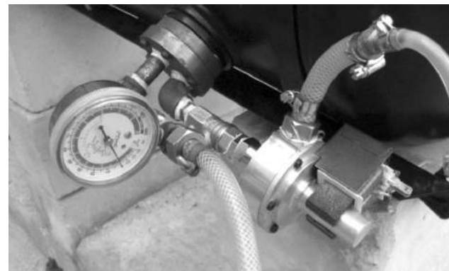
Figure 2 - Pump Connected Directly to Tank Outlet
