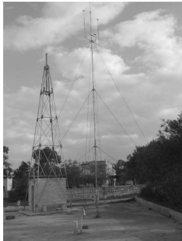
Figure 1: Lattice Tower and Wind Monitoring Mast
