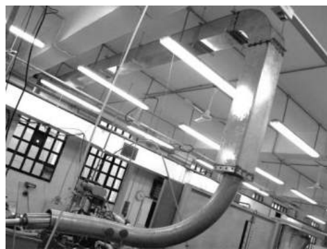
Figure 1: Complete Ducting system
