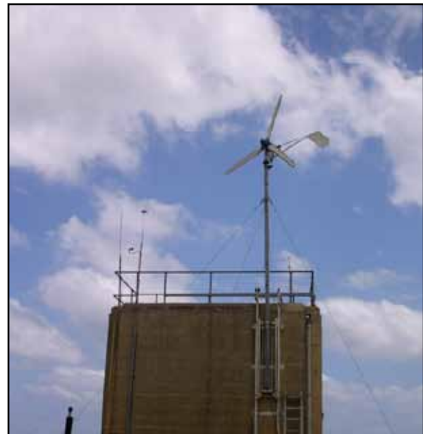
The Micro Wind Turbine installed on the roof of the Faculty of Engineering
